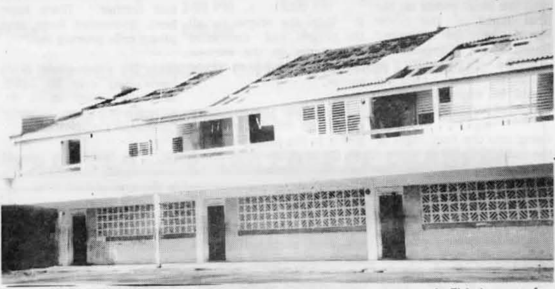
The Basseterre Junior High School, with severely damaged roof. This is one of the many schools adversely affected by Hurricane Luis.
